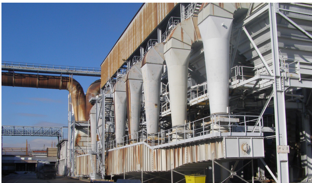
Figure 1. Gas treatment centre - FC1.
